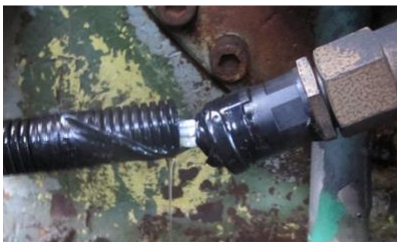
Figure 1. Example of an oil leak inside a sensor as a result of insufficient oil barriers.
